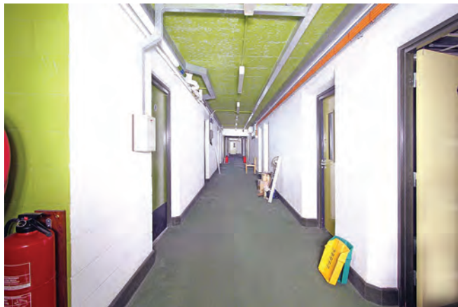
The central corridor on the upper level looking towards the main entrance. The emergency exit is to the left. The door at the end of the corridor is the upper level plant room
